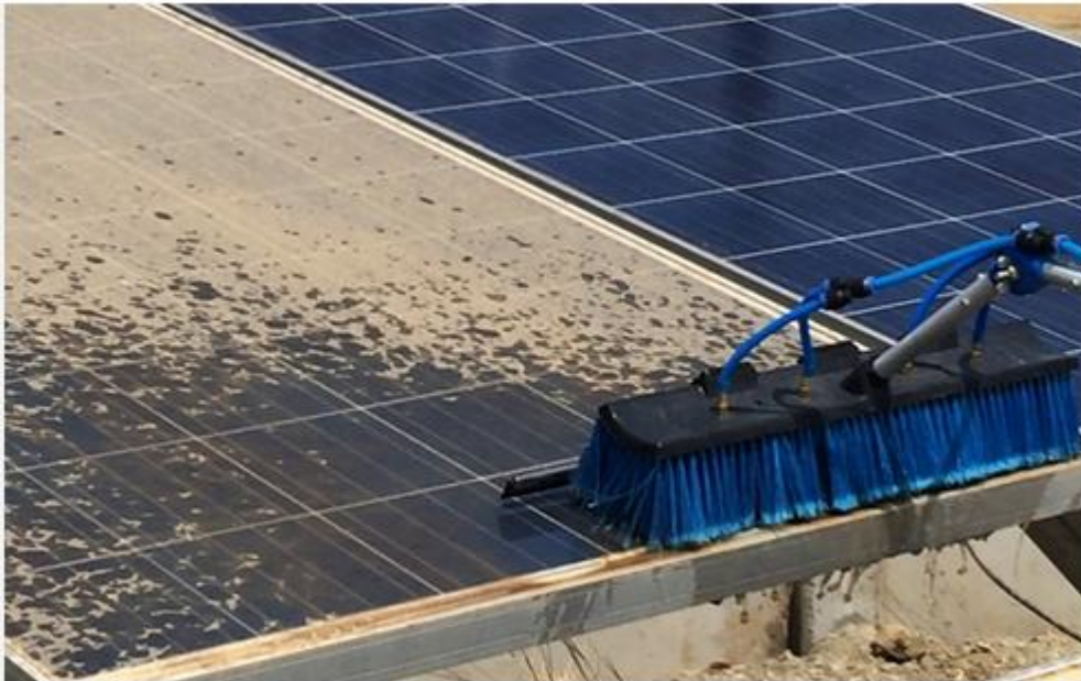
Figure 9. Dusty and Weathered Solar Panel Array. Source: https://cleanenergy4africa.org/solar-energy-and-dust-control/
